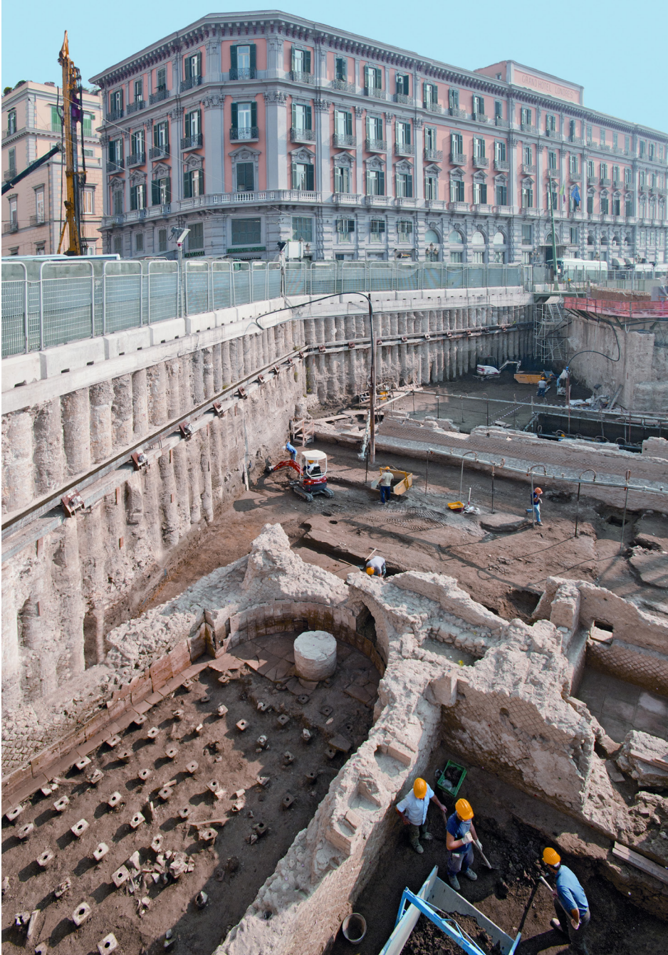
Fig. 3. The excavation site in Piazza Municipio, Naples, during metro constructions works. (Photo: ©Pierre Buch).
