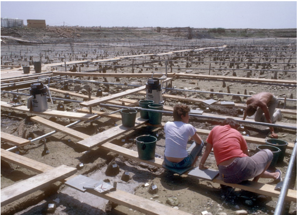
Fig. 3. The excavations of the site of Hauterive/Champréveyres (NE) in 1983, during the construction of the Motorway A5 (Photography: Éric Gentil, Laténium).
