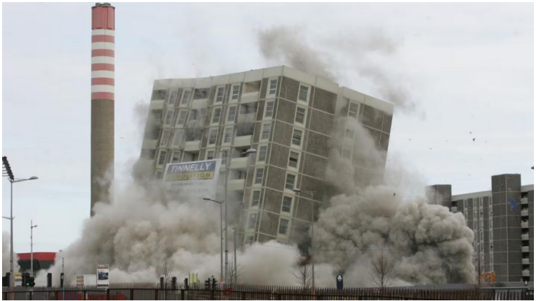
Figure 19: Demolition of McDermott Tower, 2005 (Photo: Alan Betson, The Irish Times). Available from: https://www.irishtimes.com/life-and-style/people/ballymun-at-50-from-high-hopes-to-sink-estate-1.2731512
